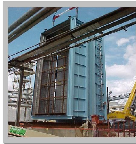
SCR Retrofit for Gulf Coast Refinery Cogen
