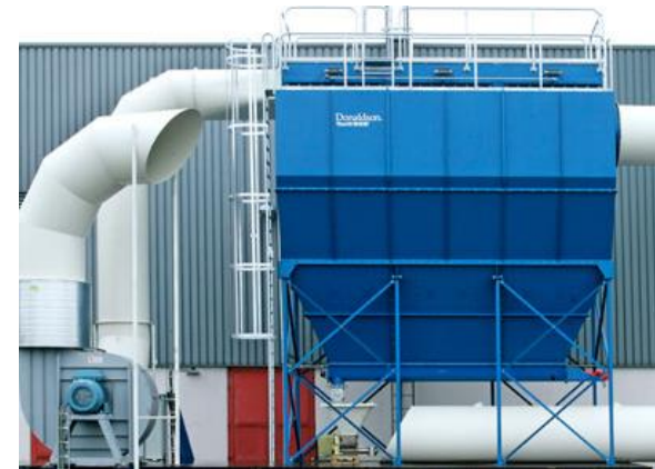
Location of leaking filter elements in baghouse filters
