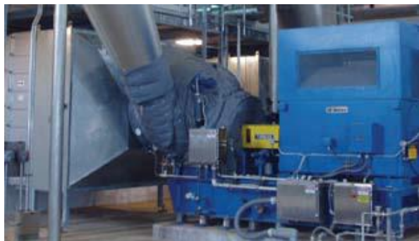
One of three Siemens Turblex KA44-GL315 flue gas desulfurization oxidation air compressors, each 18,000 scfm, 30 psig, 2500hp.
